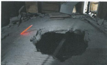
To identify a low level open edge use a red chemical light stick with a bi-pod base at ground level.
